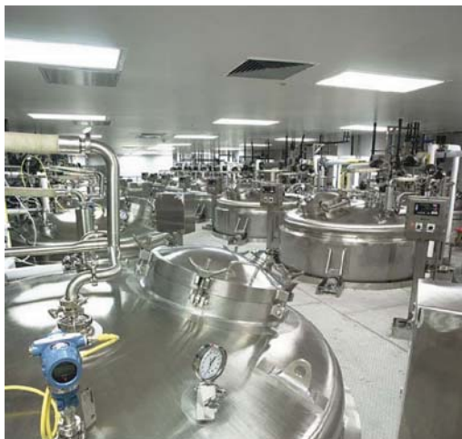
Figure 10.2 Buffer tanks and plant space requirement in a typical biotech facility.
